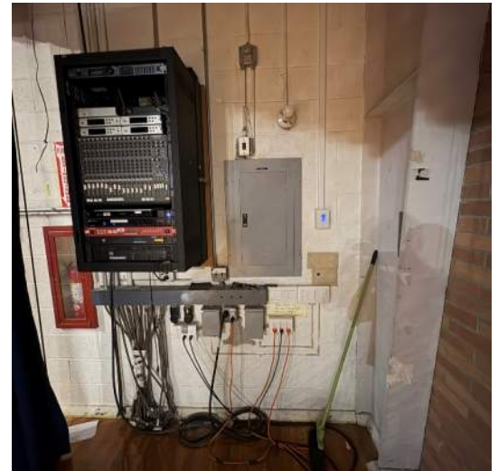
Existing stage right audiovisual equipment rack
