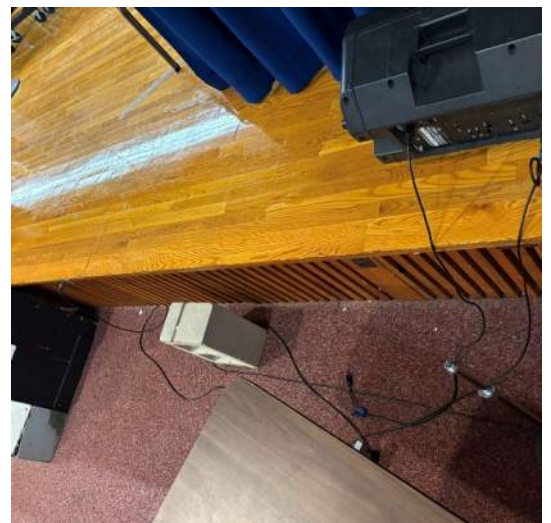
Existing stage monitor and cabling
