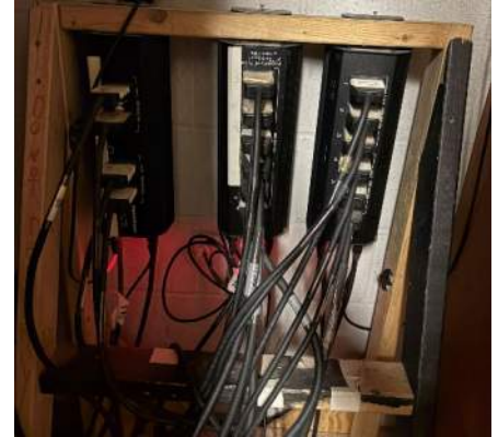
Temporary dimming packs mounted in a closet
