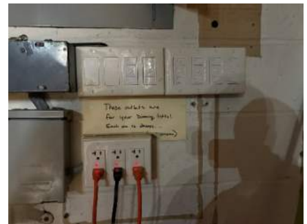
House light controls
